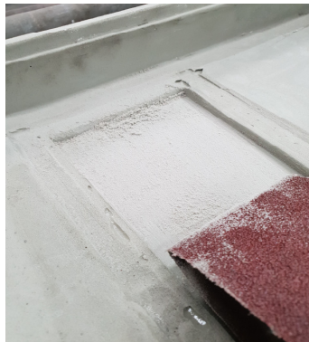
Light sanding will be required to ensure a flush fit of the flashing to the base
