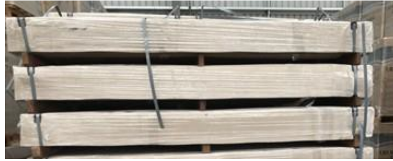
Two pieces of timber have been glued together and used as a bearer. These often break apart during handling.
